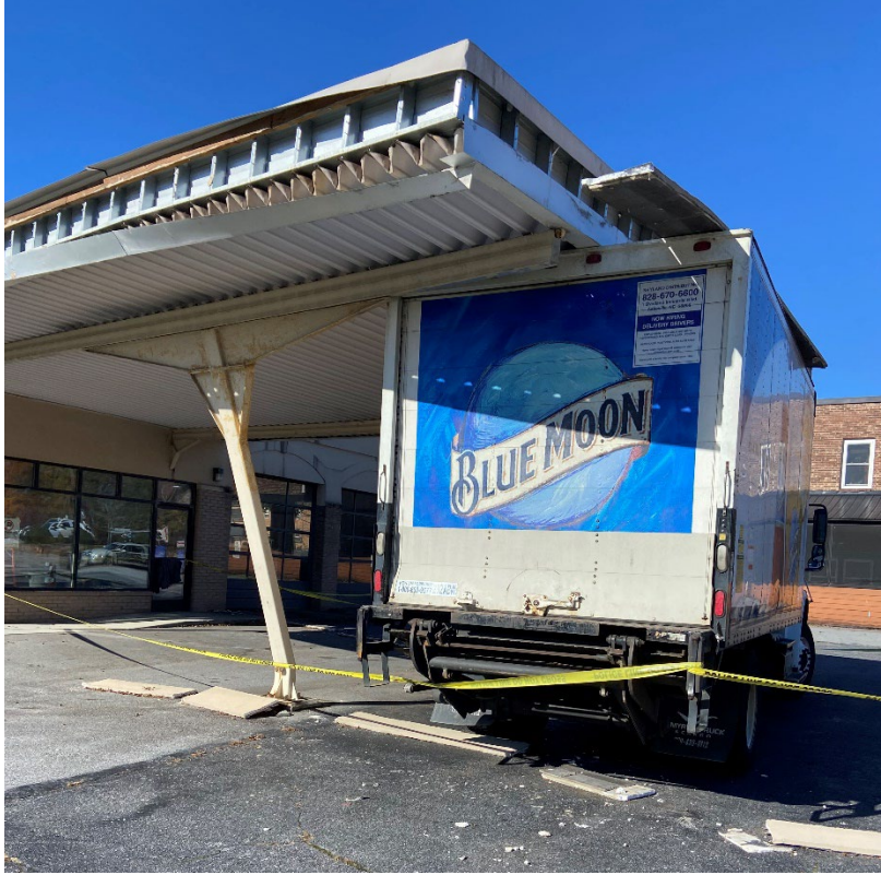
3. Former Canopy (damaged by delivery vehicle and removed)
