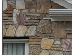
Rough cut river rock veneer with irregular courses
