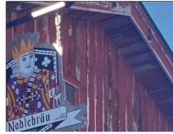
Painted board and batten siding that is weathered
