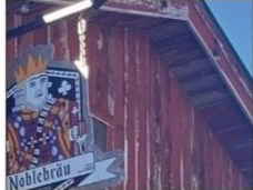
Painted board and batten siding that is weathered
