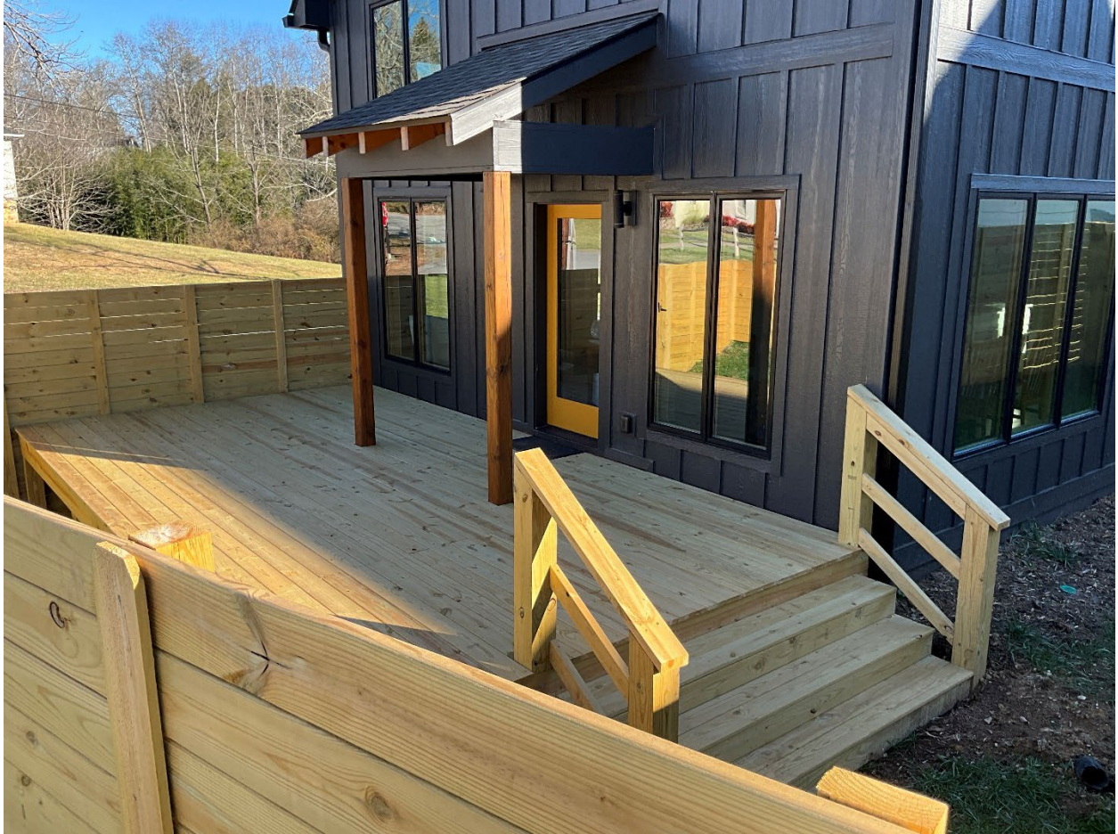
Pic 2- New deck and fence built without permits, deck does not meet setbacks.
