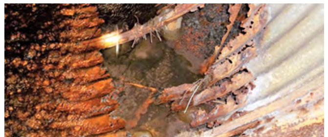
Pipe Structural Failure
