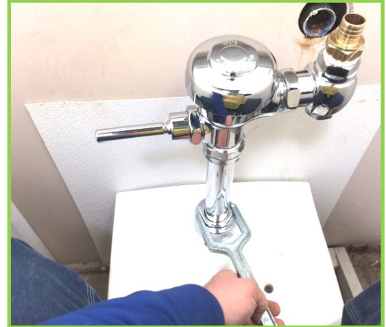
Franklin Park plumbing installations.
