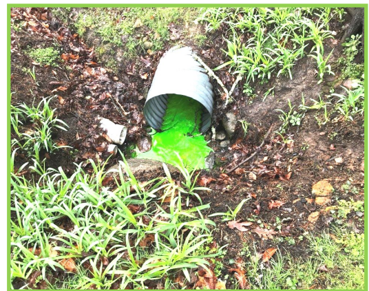
Ditch behind St. Philip's church running freely with dye.
