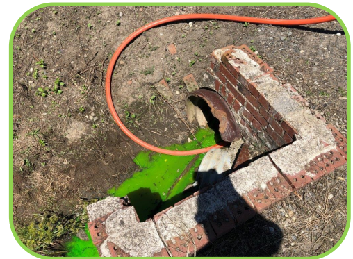
Dye reveals a plugged and abandoned drain discovered on Railroad Avenue.
