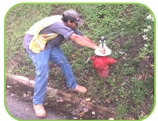
Attempt to adjust valve on fire hydrant #30-05 found inoperable.
