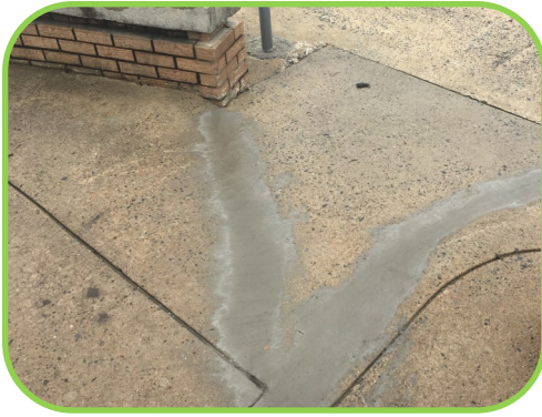
W. Main Street sidewalk crack sealed with hydraulic cement.
