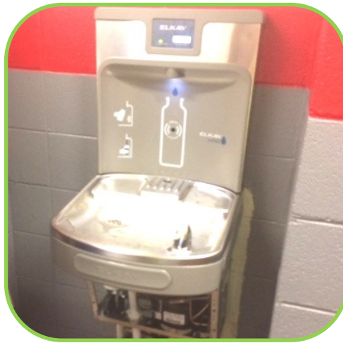
Fire Department fountain with bottle filling feature.
