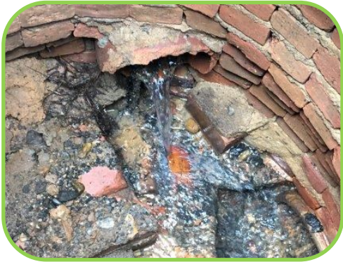
Park Avenue water leak infiltrating manhole #KC-045 prior to repair.
