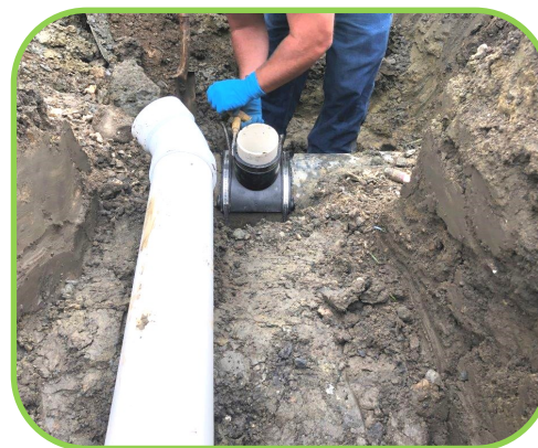
Depot service line connected to sewer main with 4" rubber saddle.
