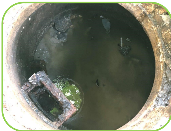
Hospital Drive manhole #LS-070 with Discovered grease blockage.
